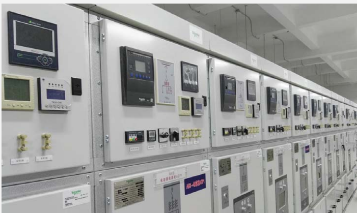
The energy for the data center is distributed over more than 50 switch-gear controlled circuits in the medium and low voltage domains .
