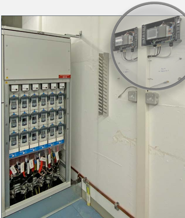
Representation of the switchgear and the decentrally mounted LINAX® PQ5000CL base stations
