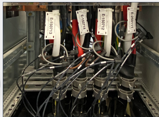
Installed Current Link modules per feeder
